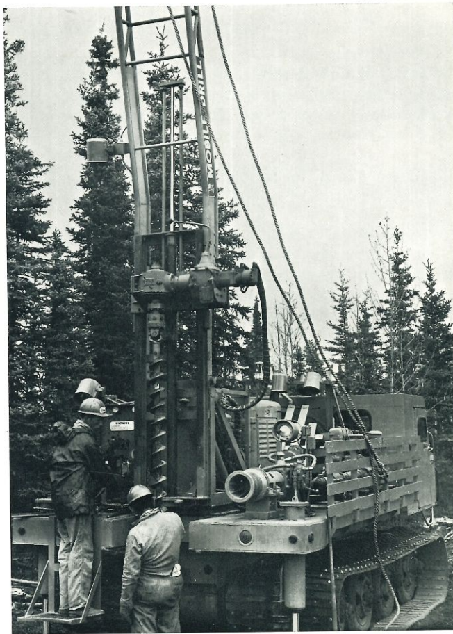
Mounted on a crawler chassis this B-40 auger rig performs penetration tests at bottom of a pre-augered vertical hole. This rig can drill holes at any angle to the surface to a depth of 30 m (90 ft) using 609 mm (24 in) augers.
